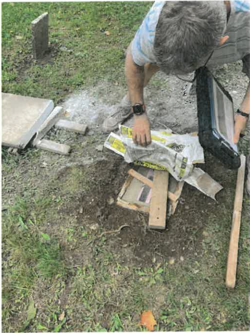
Martin Johnson from Monument Conservation Collaborative works on a new base September, 2021..
