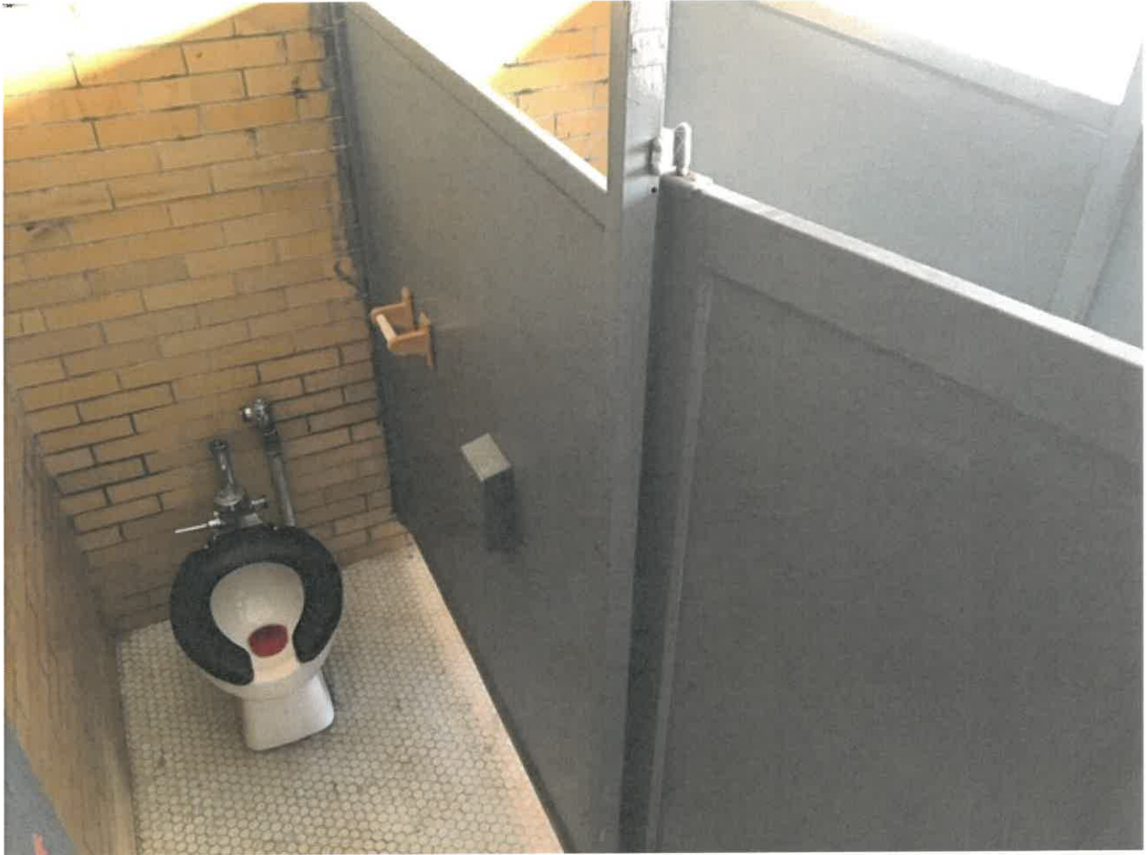
The current women's restroom has 2 stalls, and would be converted to one handicapped stall.
