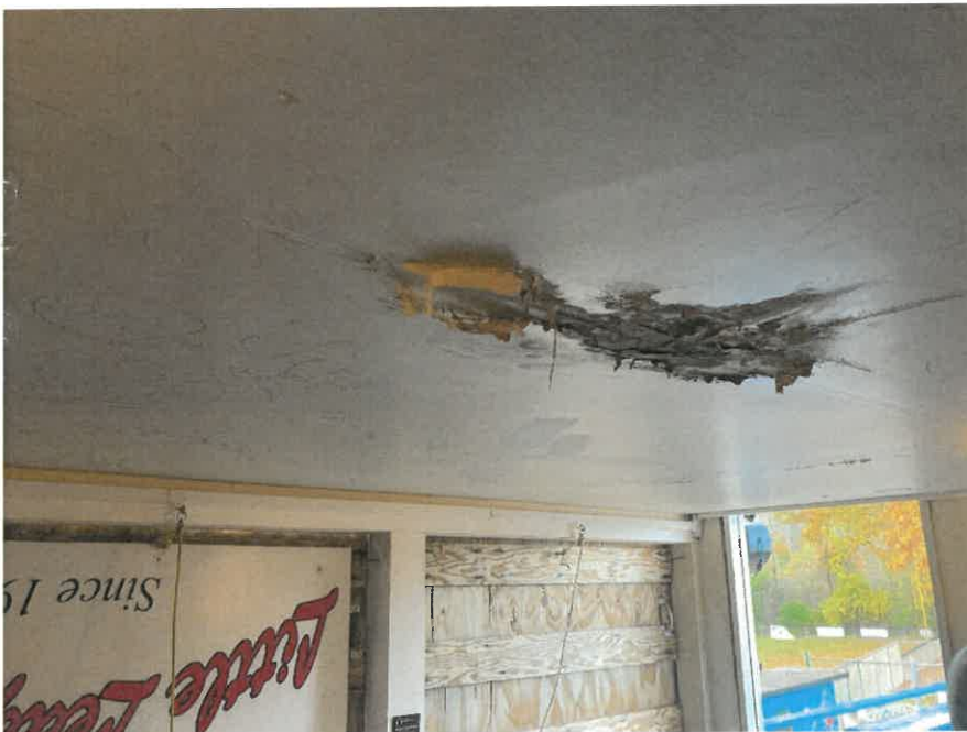
Interior scoreroom ceiling water damage.
