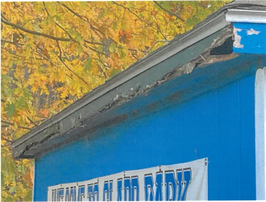
A close-up of the damage to the fascia boards.
