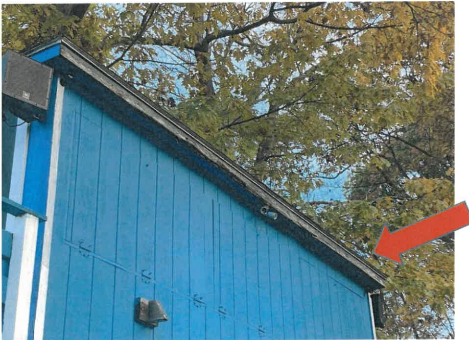
Opposite side of building with more rotting fascia board.
