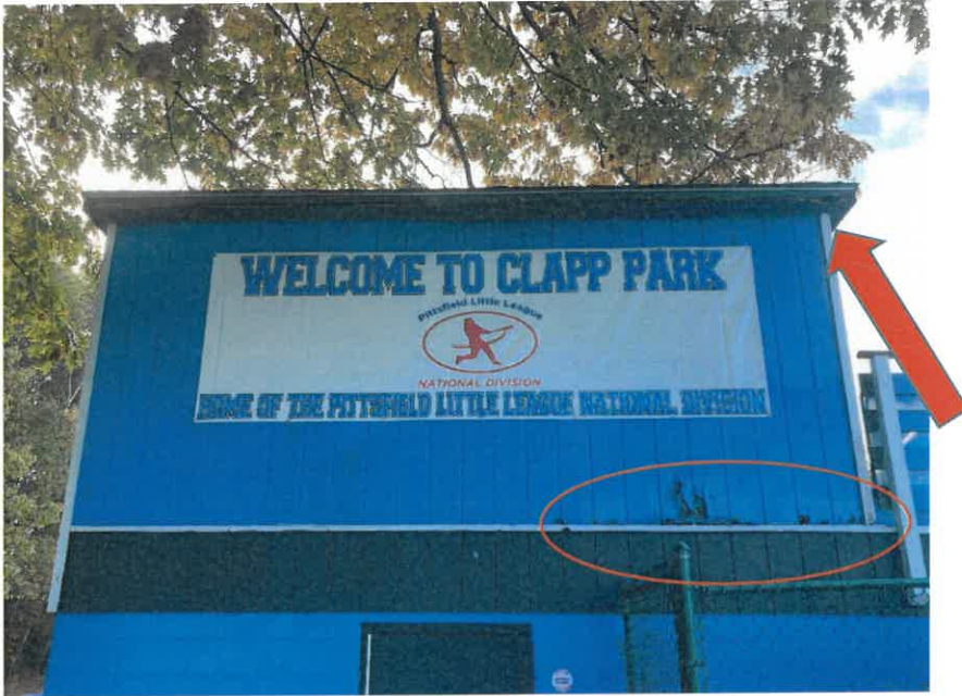
The Little League building at Clapp Park. Note the deteriorating fascia boards at the roof line and the weathered exterior siding.
